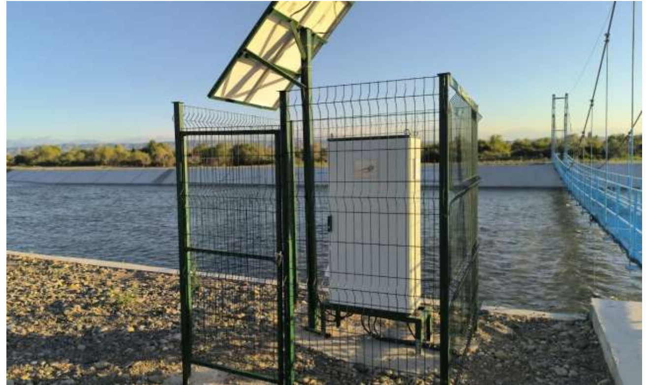
Figure 2. Arrangement of the flow meters on the Talas River
